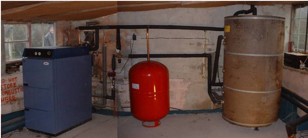
A 50kW log batch burner on left and accumulator on right.
